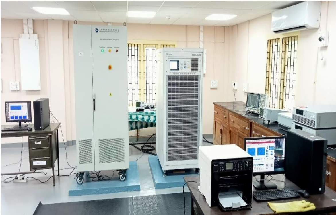
Solar Inverter Test Facility at CRTDH Chennai
