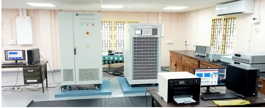
Solar Inverter Test Facility at CRTDH Chennai
