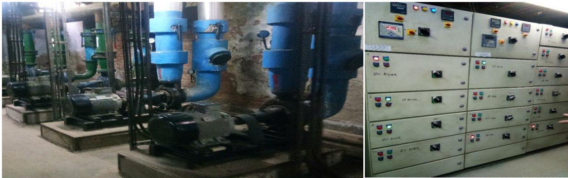
Typical view of centralized AC system and electrical panels at CSIR-IGIB, New Delhi
